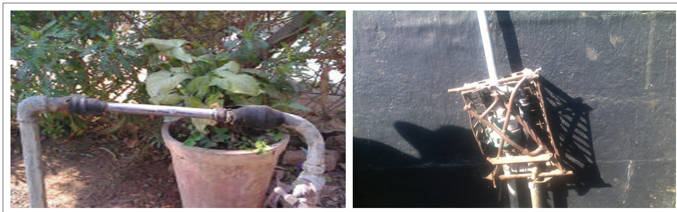
FIGURE 2: Evidence of illegal connection and meter by-passing in Chitungwiza.
